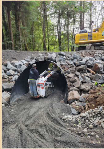
Crew from Carmesin Construction adding gravel to create a simulated stream channel inside the culvert.
