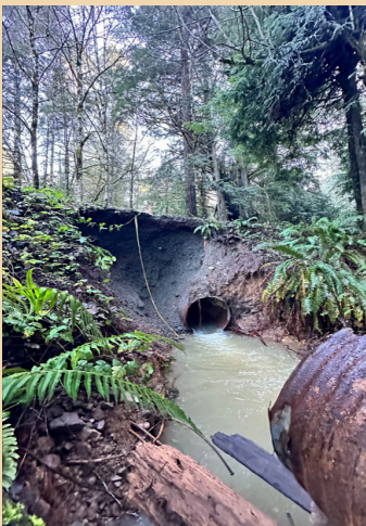
This "Before" photo shows the old culvert and erosion damage from the January 2024 storm.
